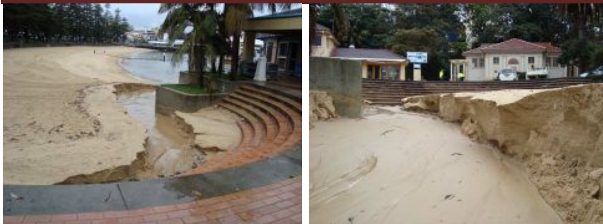
Figures 6.5c and 6.5d – Excessive scouring of the beach to the west of Manly Cove West Beach
