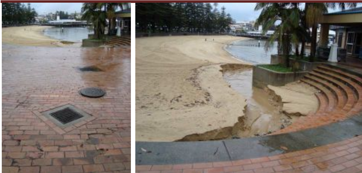
Figures 10.4.2 b & c – Scour of Manly Cove West Beach due to under-capacity stormwater system
