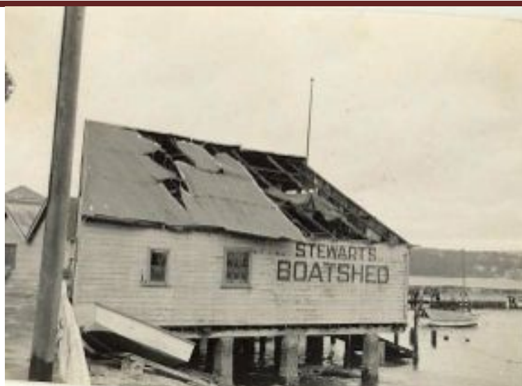
Figure 9.4.2 - Damage to Stewarts Boat Shed (Manly Launch Club) following 1974 storms
